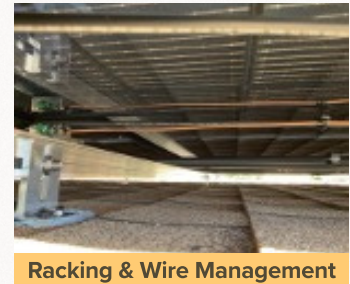
Racking & Wire Management
